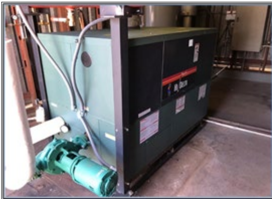
6386 Alvarado Court new boiler
