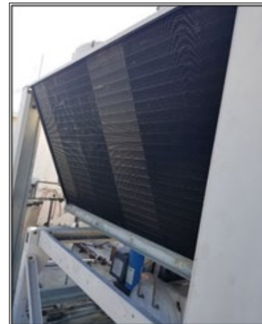
6386 Alvarado Court New chiller coils
